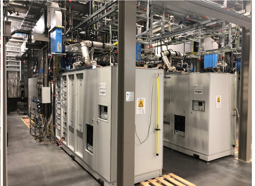
Klystrons based RF stations in Elliptical Section Modulators designed at ESS and provide in kind from ESS-BI
