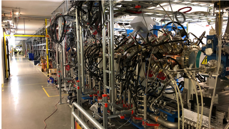
Parts of Normal Conducting Linac Under commissioning
