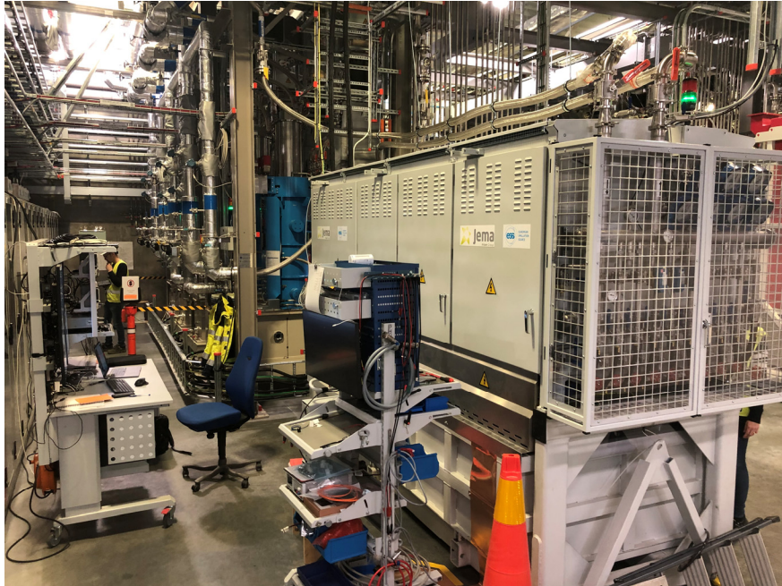
Tetrode RF Power stations in Spoke Section Tetrode RFPs provided in kind from Elettra
