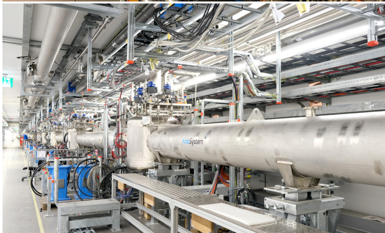
Cryo Distribution Line testing upcoming this Autumn, followed by cryomodule installation
