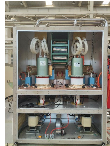
Two-TH558-tube amplifier cabinet
