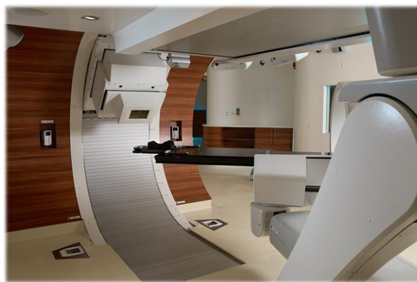
Figure 7: Gantry room: automatic patient positioning system and rolling floor. Gantry at 60°, beam entry from left.
