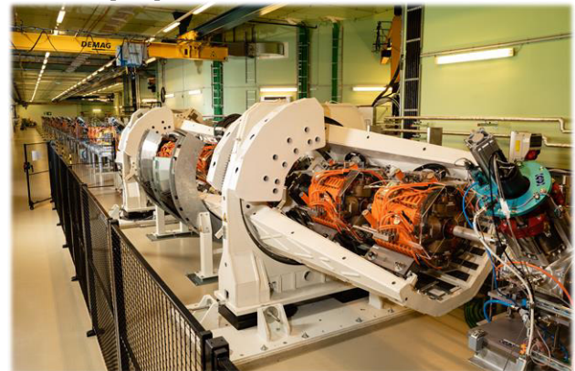
Figure 2: World-wide first rotator system (white structure) in the high energy beam transfer line. Seven quadrupoles (orange) are mounted on the structure and rotated synchronously with the gantry located downstream. With a rotator, the beam parameters at the gantry isocenter become independent from the gantry rotation angle.
